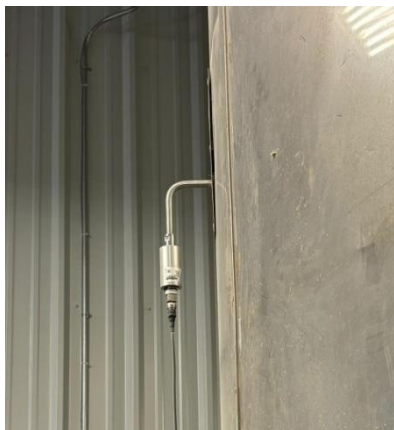
Figure 2: Ultrasonic converter on the spray dryer
