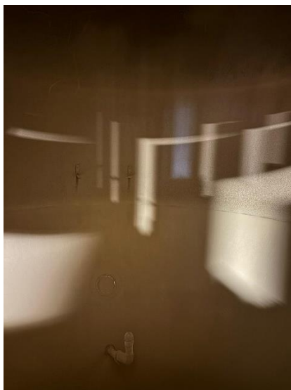
Figure 4: Seamless walls inside the spray dryer
